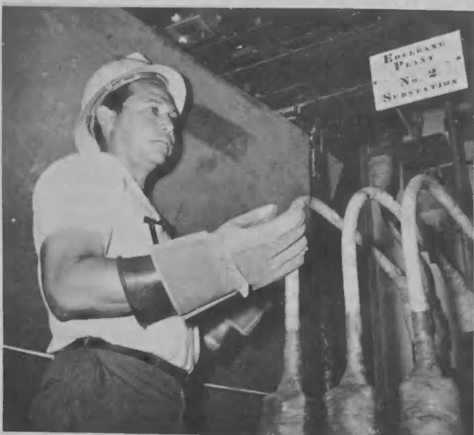
WHEN WORKING on high voltage equipment or lines, rubber and leather gloves are used. ORA TA traha ariba equipo of linja di alta voltahe, handschoen di rubber y cuero ta ser usa.
